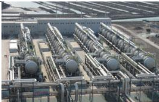
IDE's installation in Tianjin
